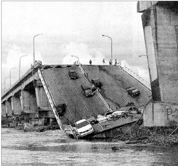
The Kaohsiung-Pingtung bridge, which collapsed yesterday
